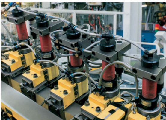
Stamping units placed in line
